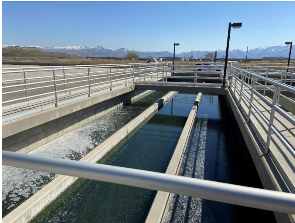
Figure 3-10 Chlorine Contact Basin
