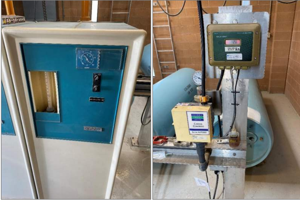
Figure 3-11 Chlorinator, Storage Tanks, and Scale
