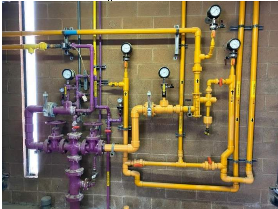
Figure 3-12 Existing Unused Chlorine Feed
